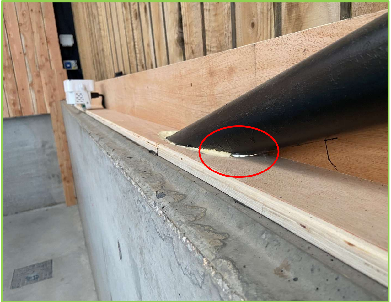
Drawing 14: Gaps in junction between wood and frame.
